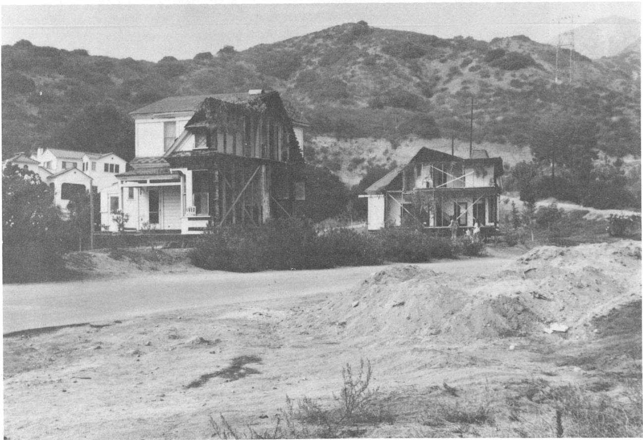
The two sections of the Doctors' House rest expectantly adjacent to their new foundations prepared in Glendale's scenic Brand Park. The future is here for this historic relic from the city's past. (Photo by R.M. Newcomb)
