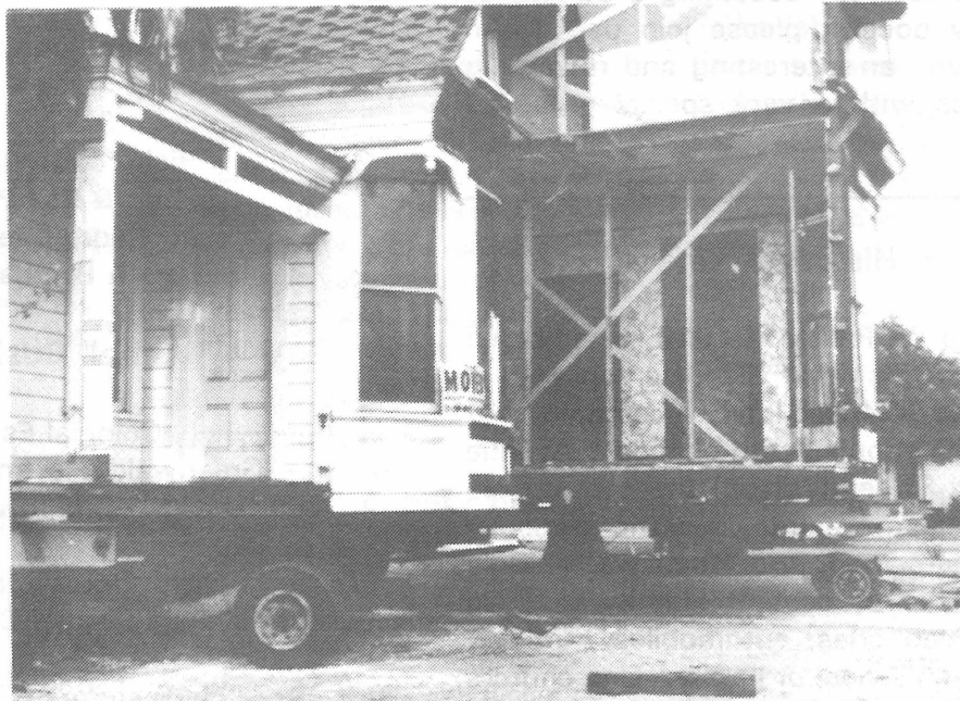
The Doctors' House poised for the move. The Glendale Historical Society worked hard to keep vandals at bay and to salvage as much as possible from the building and the site. (Photo by R.M. Newcomb)
