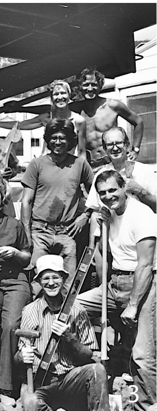
House was restored, volunteer Marie Luft for their heroic square headed nail found in Marie's discarded work shoes
