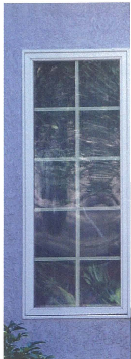
An unsightly vinyl replacement of the glass and the lack of muntins. These windows ruin the property.
