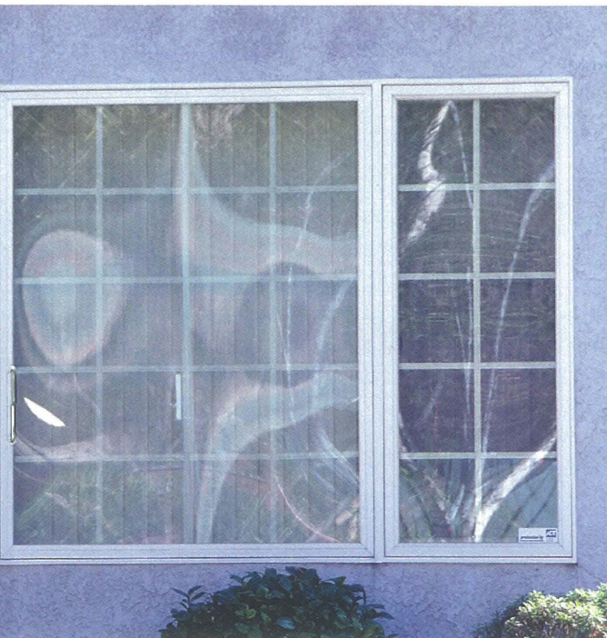
Replacement window with interior muntins (dividers). Notice the warp of shadowing that would be created by original wood windows. Lack of character, do not fit the style of the home and devalue
