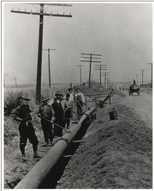
San Fernando Road, ca. 1906: Installing gas pipeline PHOTO: Special Collections, Glendale Library
